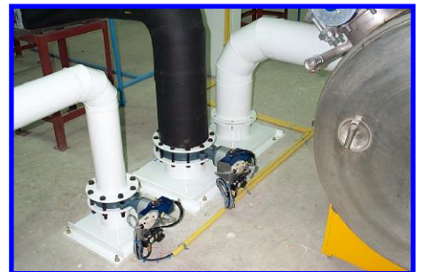
BSL3+ and BSL4 laboratories: Process Engineering, AHU system, including detail engineering, turn key plants.
