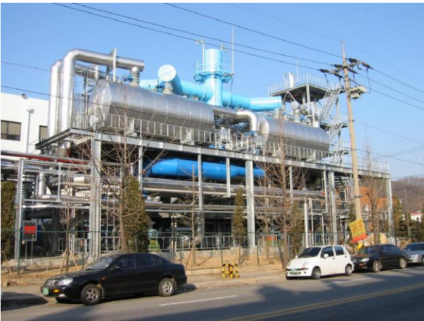
Solvent Recovery Plant in South Korea
